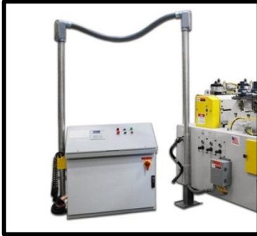
Overhead cable run
