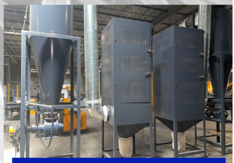
(2) Baghouse Dust Collectors
