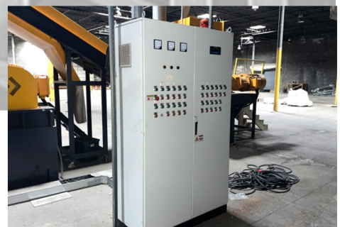
Integrated Control Cabinet
