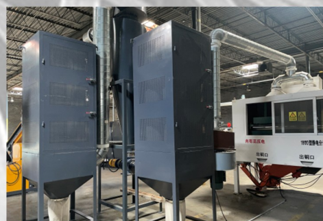
(2) Baghouse Dust Collectors
