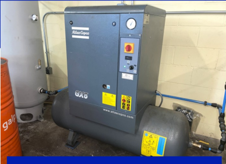
2014 - Atlas Copco Compressor
