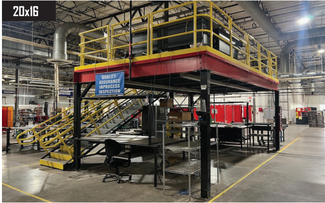
Mezzanine 20' x 16' with Stairs, Lights and Power.
